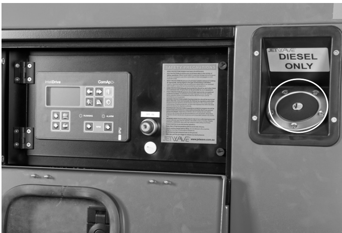
Figure.5 - Diesel fuel supply tank
